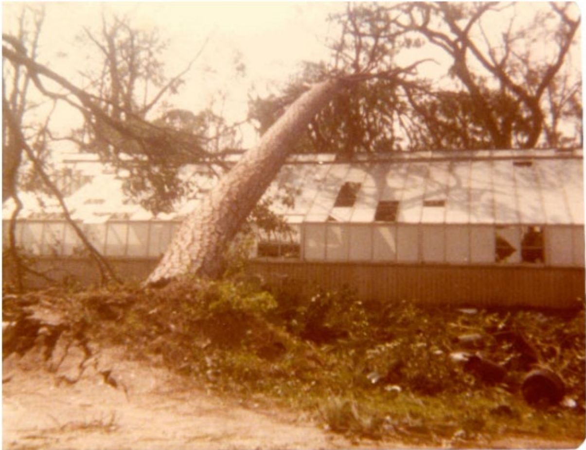
The Conservatory after Hurricane Frederic—damaged but still sheltering my dad’s beloved orchids.
